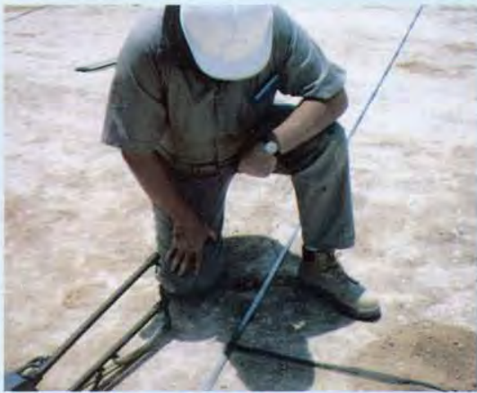
Mixed Metal Oxide tank base Grid System-connection between anode and conductor bar
