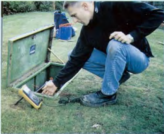
Monitoring an underground tank CP system
