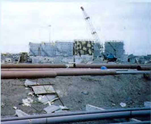
Corrpro Tank Grid CP Systems were installed on all tank bases at Reliance, Jamnager
