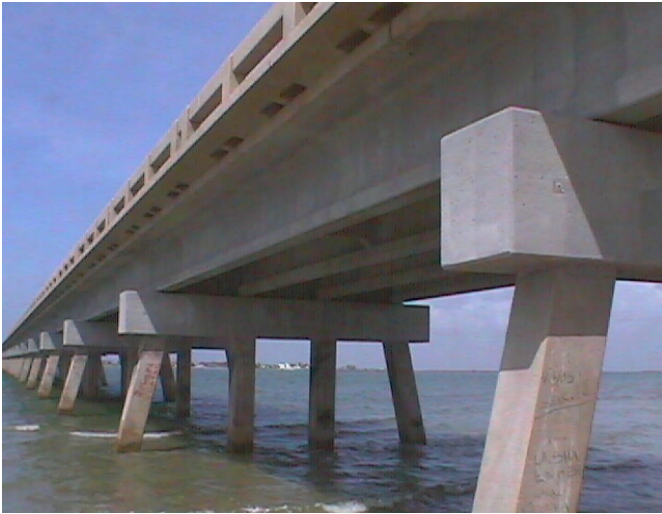
Figure 8. Thermally sprayed Al-Zn-In anode for galvanic cathodic protection of a concrete bridge.
