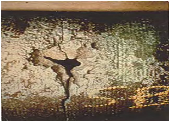
Figure 1 Fracture of Cast Iron Pipe Weakened by Corrosion
