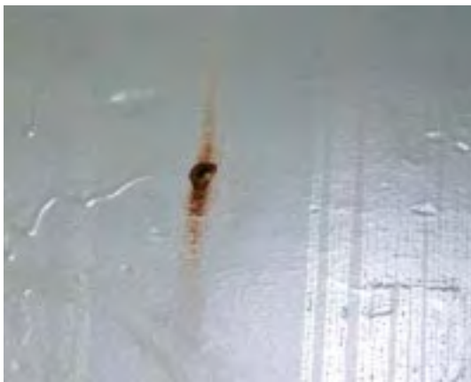
FIGURE 4 Penetration of Tank by Pitting Corrosion
