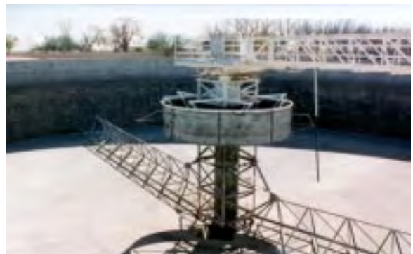
Figure 2 Water Treatment Clarifier
