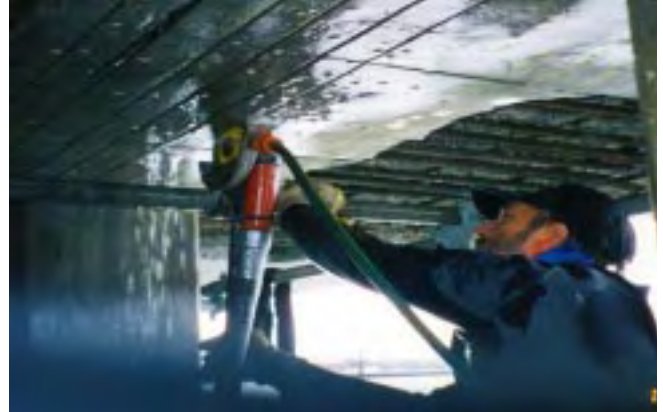
Figure VI. Slotted system installation on the underside of a wharf terminal in Australia.
