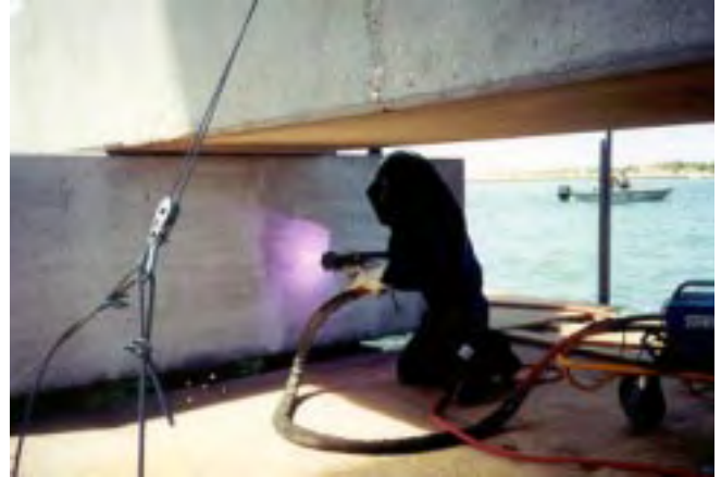
Figure VII. Arc spray application of galvanic Al-Zn-In to a bridge pier in Texas.
