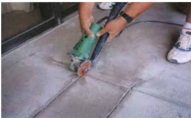
Figure V. Slotted system installation on the top side of a condominium balcony in Florida.
